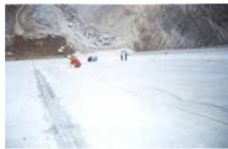
Figure 51. Gudongkou Concrete Face Rockfill Dam and construction scene of optical fiber sensors to be embedded
