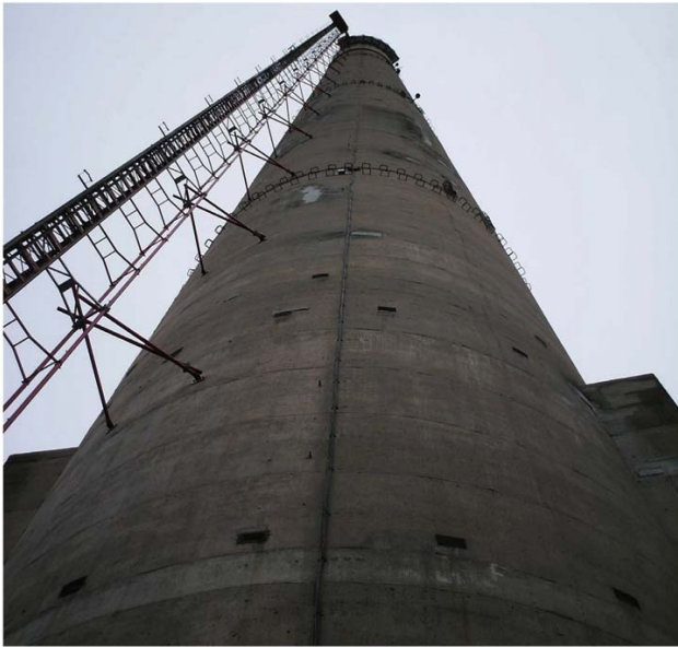
Figure 2 TMD under construction, with lower accelerometer box in position and flue openings flanking chimney
