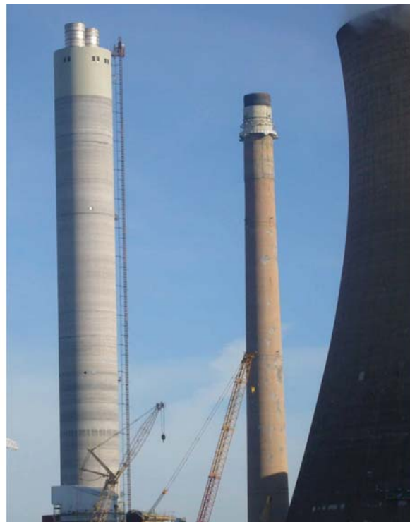
Figure 1 Chimneys at Rugeley Power station: old chimney crowned by tuned mass damper is in the centre
