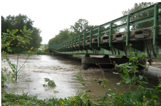
(a) Loss of Center Pier
